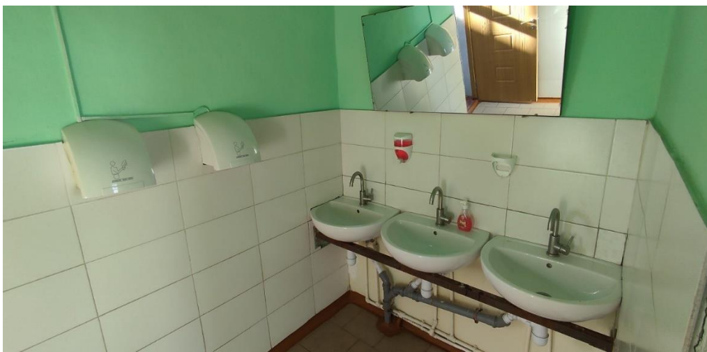
Hand washing facilities
