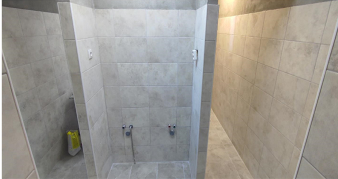
Handwashing facilities GTS common access
