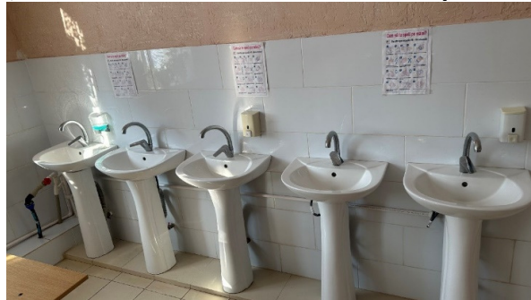
Handwashing installations inside the dining room
