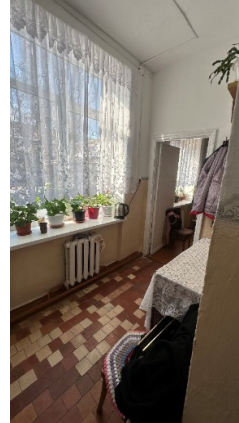
Current situation toilet for girls, level 2.
