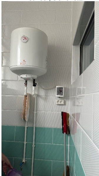
1st floor, boiler room
