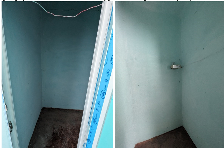
2nd floor – rehabilitation/construction of sanitary groups for teachers in the existing spaces including renewing flooring, walls, and ceilings, and ensuring that all elements meet current health, safety, and accessibility standards. Considerations should also include upgrading water supply system, sanitation system, plumbing and sewerage systems, renovating fixtures and fittings, improving ventilation, electrical system, installation of water heaters, handwashing facilities, waste management, aesthetic, and functional improvements, ensuring accessibility for persons with disabilities, and adhering to relevant building codes and regulations
