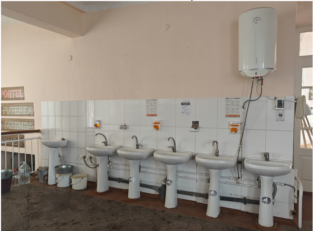
washbasins on the hallway
