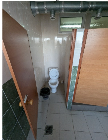
GTS girls and staff, necessary to renovate ventilation and change doors for cabins
