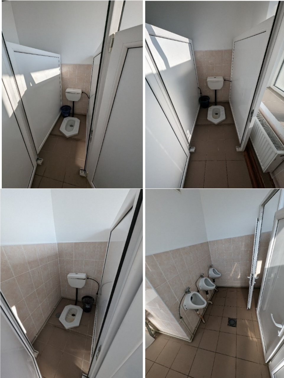
GTS boys classes 1-4 floor 1 – 3 toilet bowls, water heaters, installation of 3 urinals and separation walls, installation of 2 washbasins for small children, soap dispensers and paper holders, mirror installation
