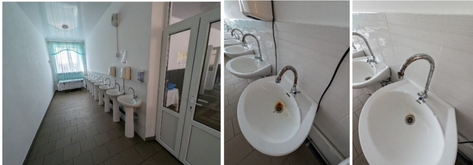
Canteen entrance – installation of 3 washbasins for small children, soap dispensers and paper holders, mirrors, water heaters, hand dryers
