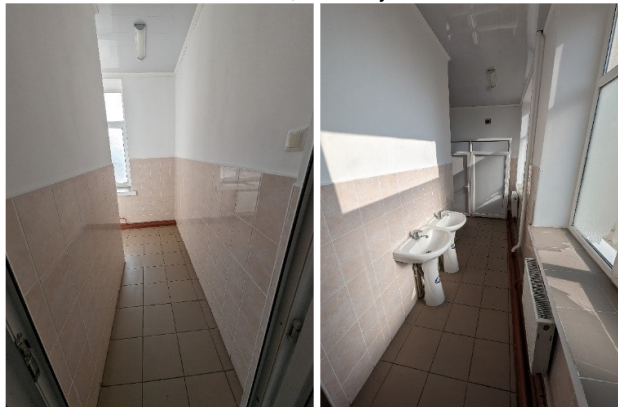
GTS boys classes 1-4 floor 1 – 3 toilet bowls, water heaters, installation of 3 urinals and separation wall, installation of 2 washbasins for small children, soap dispensers and paper holders, mirror installation
