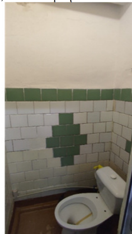
Toilet for technical staff in the canteen
