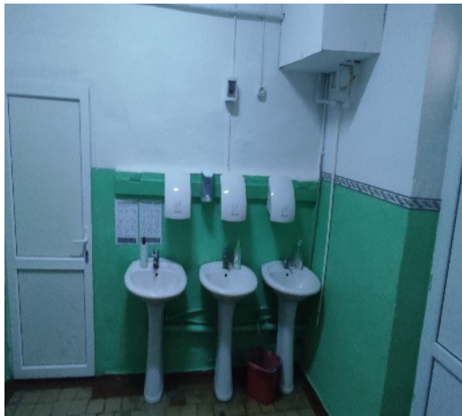
Handwashing facilities - canteen access
