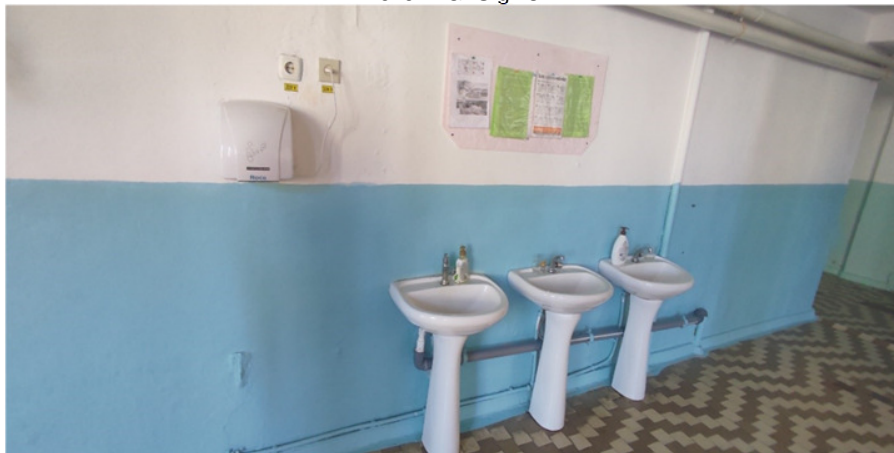
Handwashing facilities - canteen access
