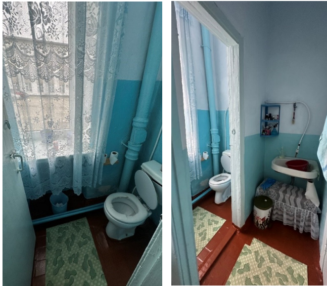
WASH facilities for kitchen staff
