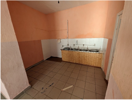
Canteen access, it is necessary to repair the ceiling, floor, tile, changed washbasins and sewage system
