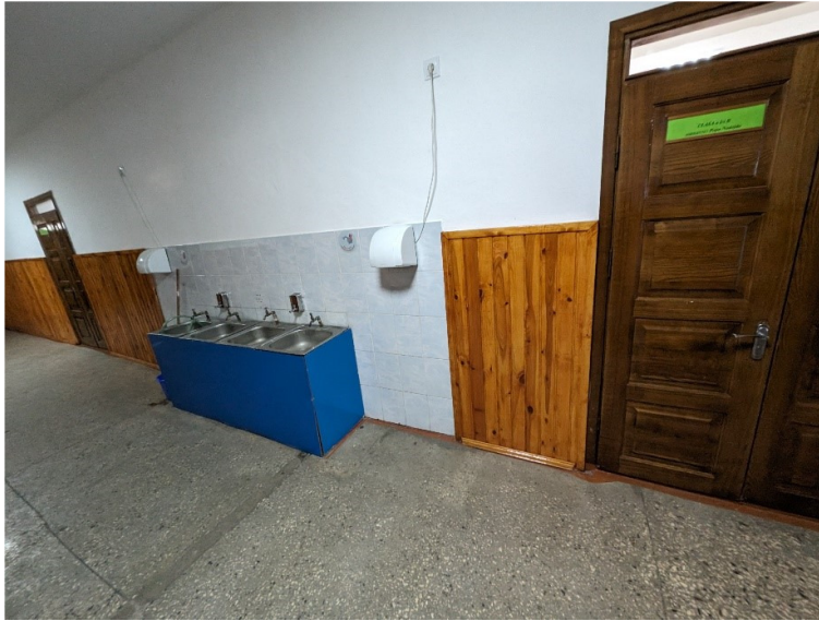
Access washbasins canteen, it is necessary to repair and change washbasins
