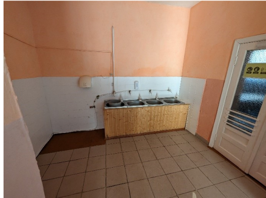
Canteen access, it is necessary to repair the ceiling, floor, tile, changed washbasins and sewage system
