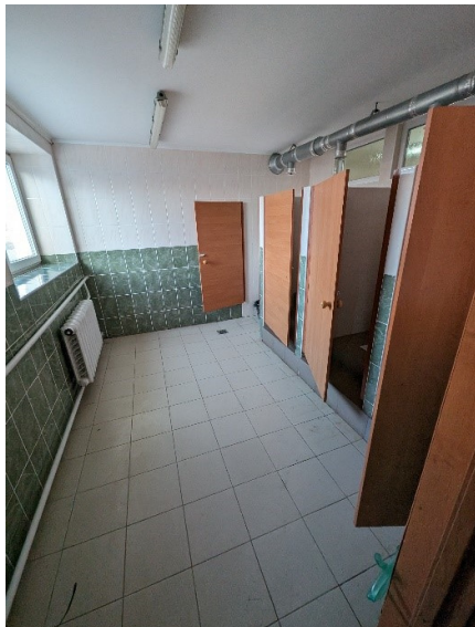
GTS girls and staff, necessary to renovate ventilation and change doors for cabins
