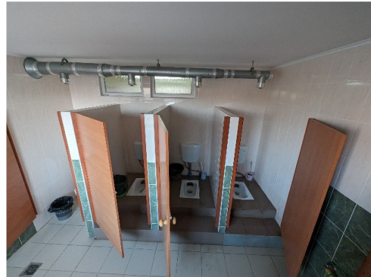
GTS girls and staff, necessary to renovate ventilation and change doors for cabins
