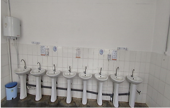
Handwashing facilities - canteen access
