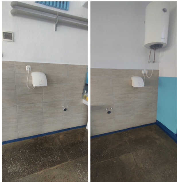
Handwashing facilities - canteen access
