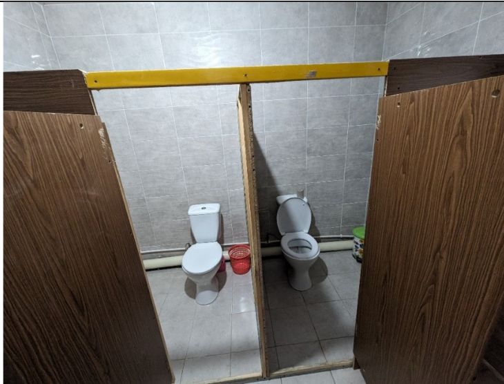
SG girls – installation of ventilation system, replacement of tap at the washbasins, modification of a cabin for menstrual hygiene for woman, installation of water heaters, paper holders and soap dispensers, mirrors, installation of separation walls for cabins (currently improvised from glued wood), installation of hand dryer
