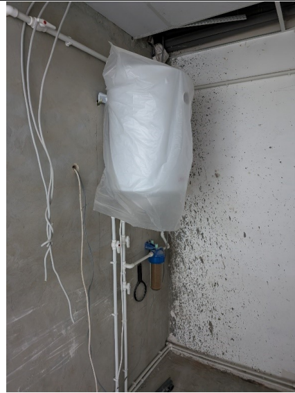
Water heater for SG installed 2022
