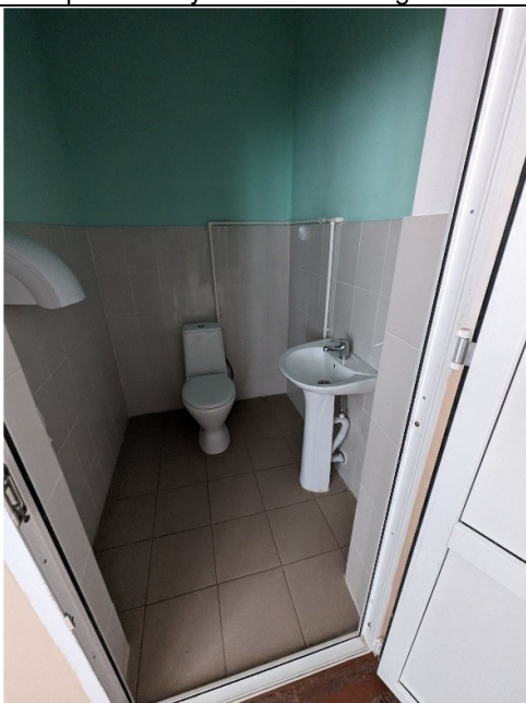
GTS staff-missing water, ventilation and lighting needs to be repaired
