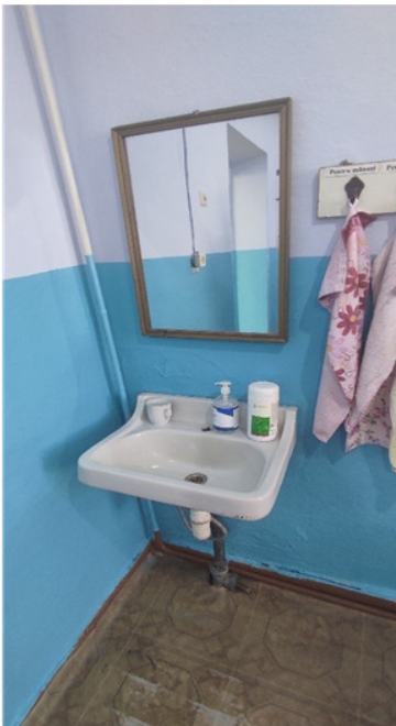
Handwashing facilities medical office
