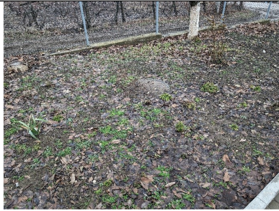
Cesspool, necessary to build the local wastewater treatment plant
