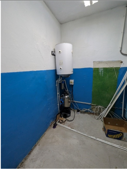
Cafeteria water heater
