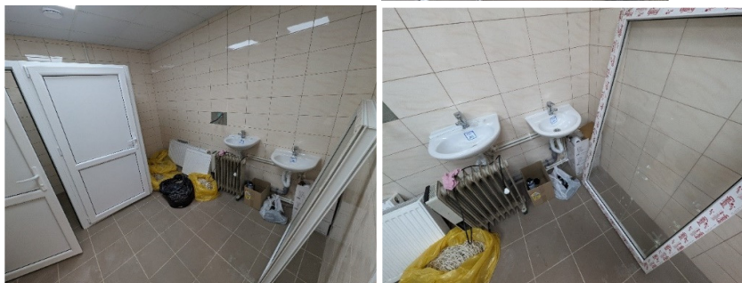
SG constructed in 2022 for persons with reduced mobility reequipment with all appropriate element as guide and support bars
