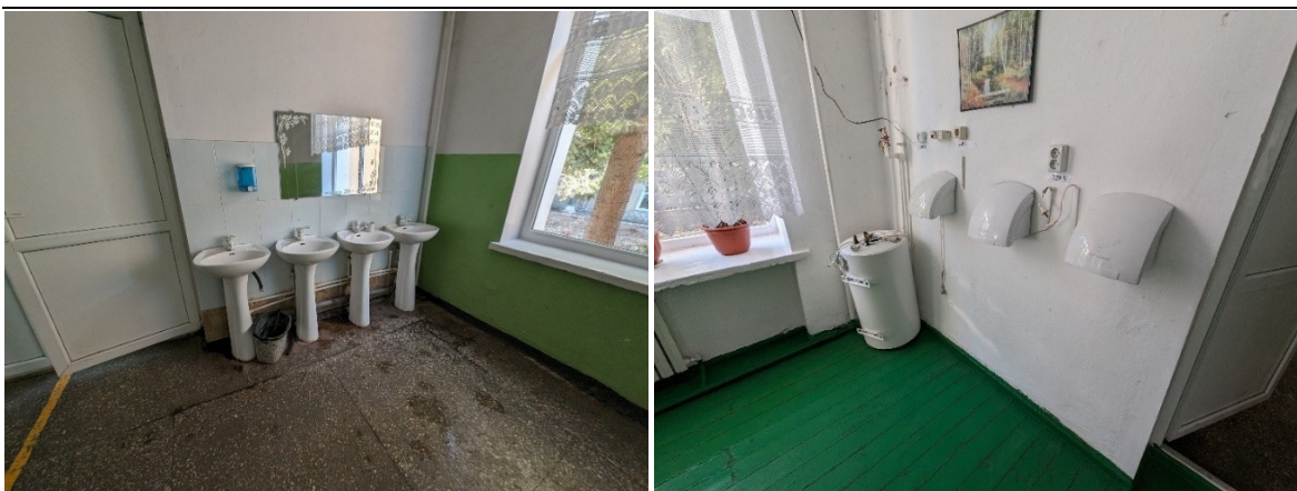
Cafeteria access – water heater replacement, mirrors installation, paper holders and soap dispensers , 2 additional washbasins for small children
