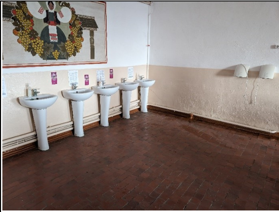
Access to the centralized water canteen pressure is poor, it is necessary to repair the access area and change washbasins
