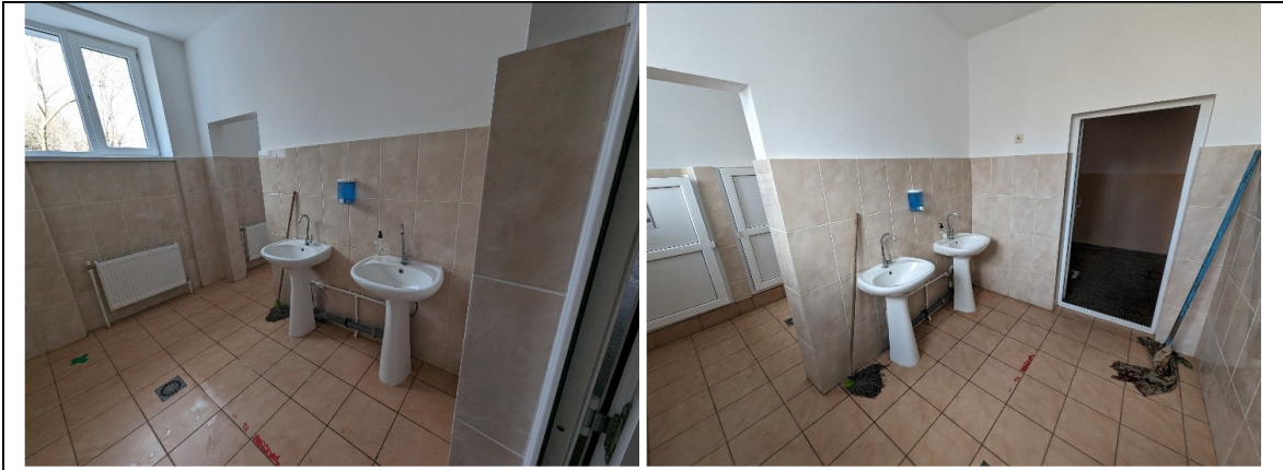
SG girls class 1-4 – paper holders and soap dispensers, tap replacement, water heaters installation, mirrors
