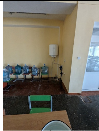
Cafeteria access water heater view
